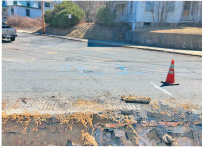
Where the pipe was found.
