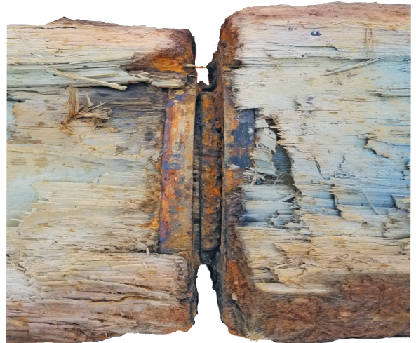
A metal coupling joins two pipes.
